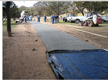
Plastic sheeting was used to cure the StoneyCrete™ for maximum strength. Pervious concrete pavement was placed right on top of the decomposed granite path.
