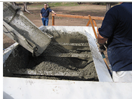
This paving machine allowed a City crew to pave nearly 1350 feet of eight-foot wide path in six and a half hours--even though they had no experience with the new paving equipment.
