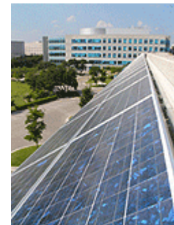
PV system installed at IBM's Tivoli complex.
