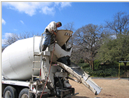
Mix truck driver inspects his load of pervious concrete at Shoal Creek Hike and Bike Trail in Austin, Texas. Seventeen loads of StoneyCrete™ pervious concrete were placed and finished in record time.
