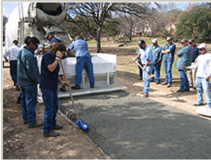
Employees from the City of Kyle look on as COA employees place nearly 80 feet of path in under ten minutes. The City of Kyle is considering installation of pervious trails.
