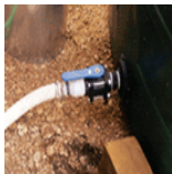
Many components of rainwater collection
