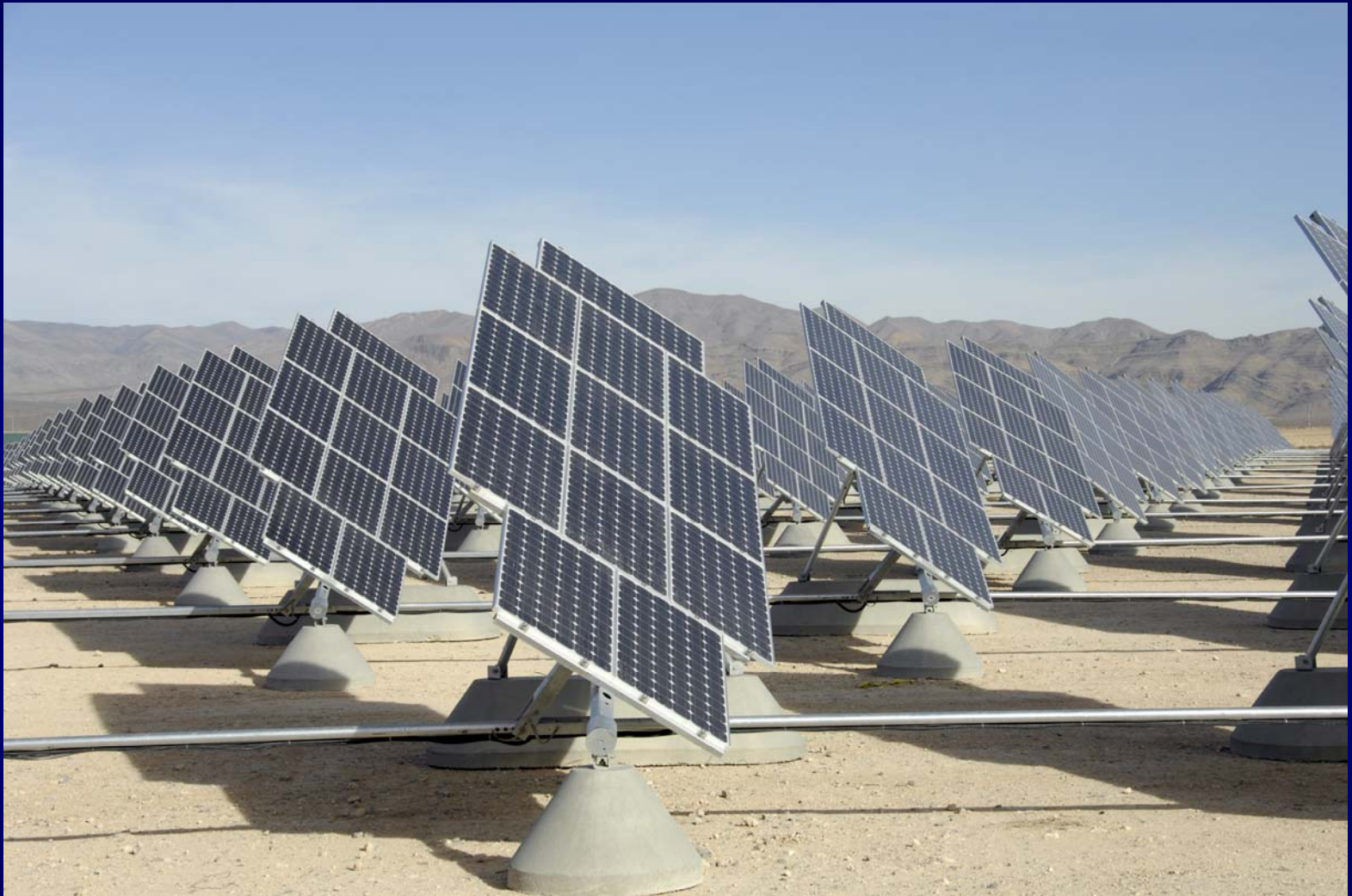
14 MW Nellis Air Force Base – Completed Dec 07
